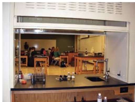
Fume hood shared by prep room and lab/classroom
