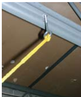
A 3/8" eyebolt is mounted to the ceiling bar joist. Tensile strength of bolt is over 1,000 pounds. The braided nylon rope has a tensile strength over 400 pounds.
