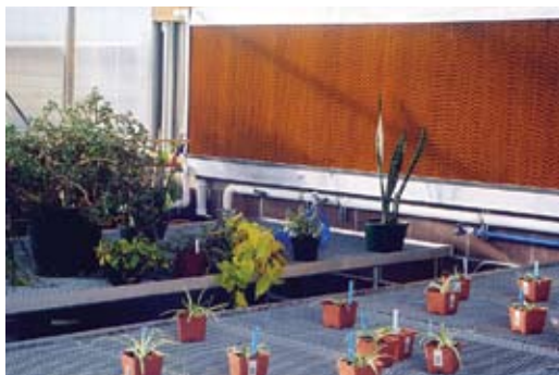
An evaporative cooler wall
