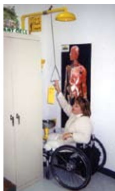
An accessible safety shower/eyewash
