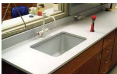
A deep perimeter sink with pull-out face shower
