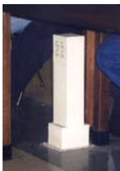
An undesired construction change
