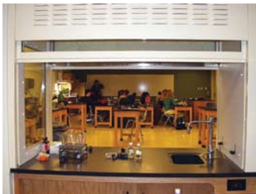
Fume hood shared between prep room and lab/classroom
