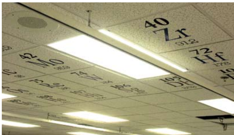
Unistrut system for suspending items below ceiling
